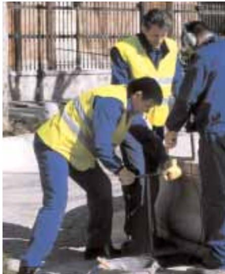
■ Drinking water and sanitation in Alcalá de Henares. Madrid
